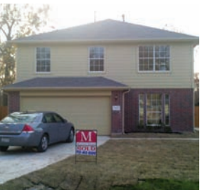
Kimm Perez visits her new home site during construction (top). It was completed in February 2010.
